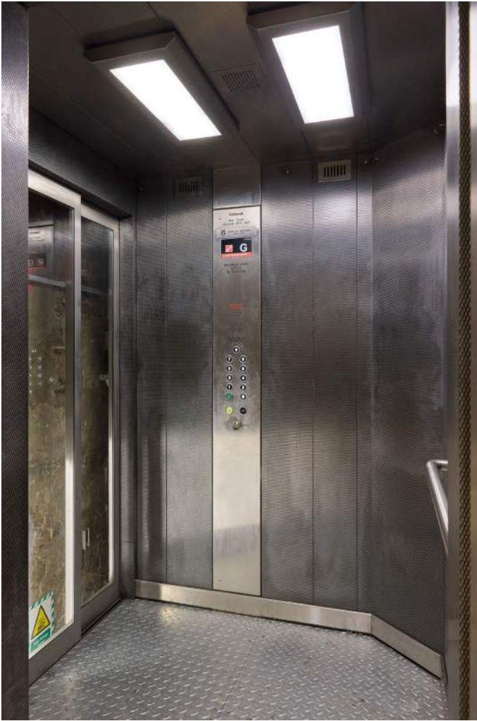
Passenger lift car with glass door to see original lift structure
