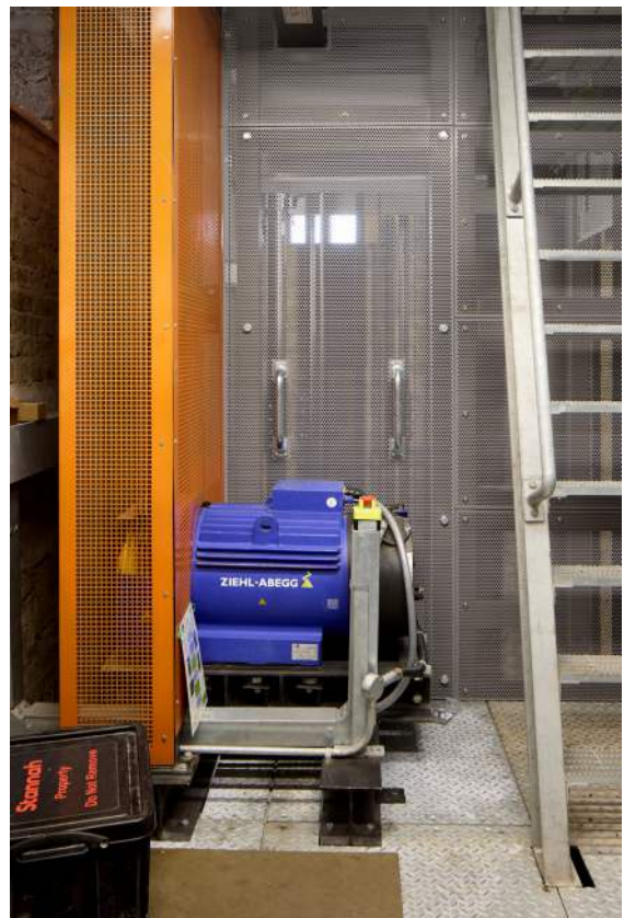
Passenger lift control room
